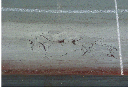
Figure 18. Zigzag cracks along the plate edge.
