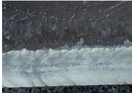
Figure 17. Typical transverse cracking.
